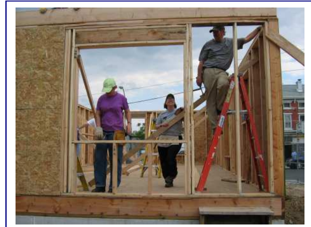
Pictured above are some of our hard working volunteers framing up some of the new homes that the Bovis Lend Lease golf outing will help to fund.
