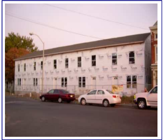
Pictured above is the current progress we have made on our five-home row house project.
